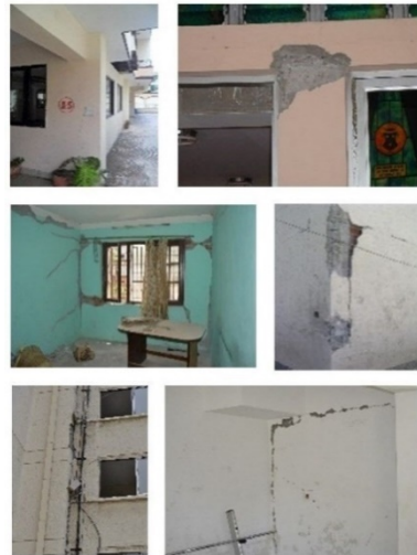
Damage on a building
