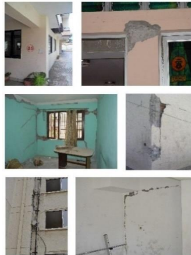
Damage on a building
