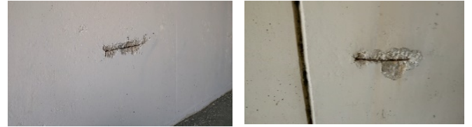
Figure 2. Defect 1 (left) and Defect 2 (right).
